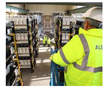
Alstom Grid UK HDVC Power Systems
